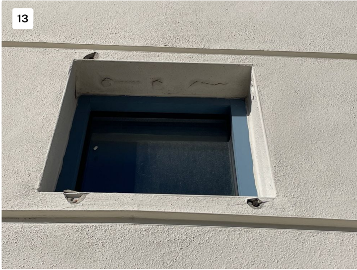
Cracking stucco around windows
