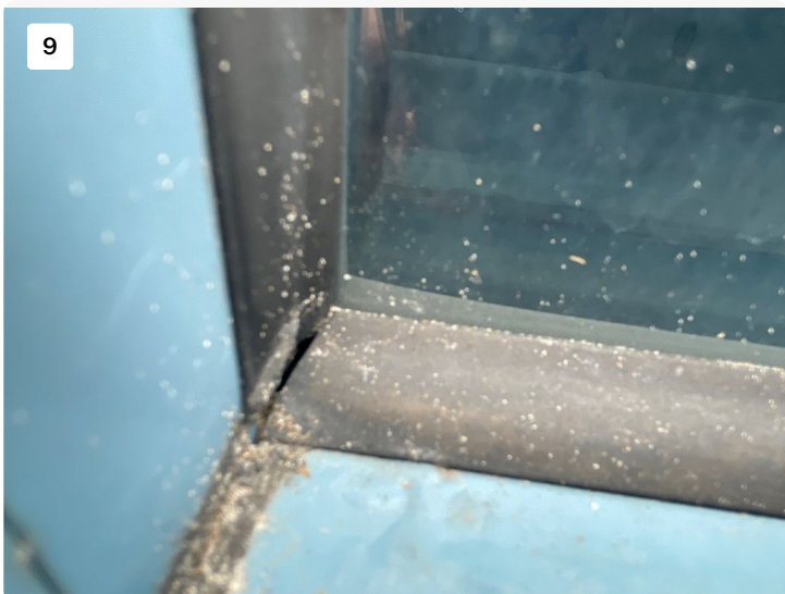
Openings at window seal corners
