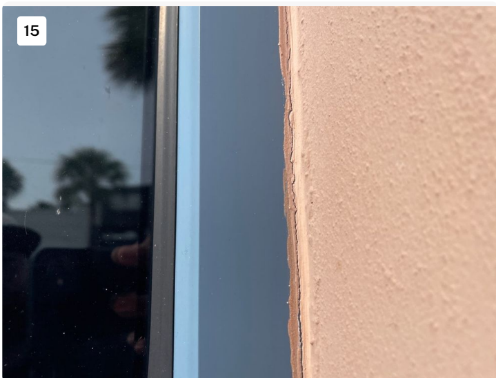
Window perimeter sealant cracking
