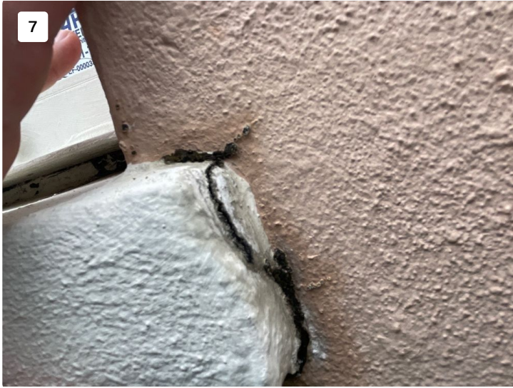
Stucco cracking at window frame
