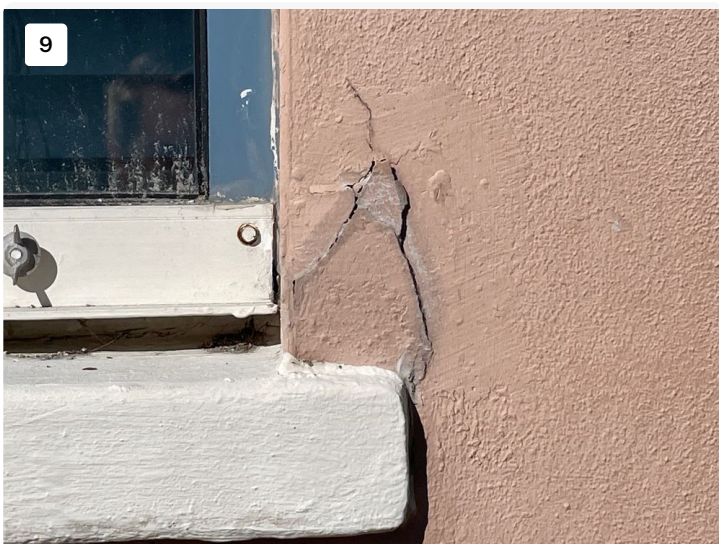
Cracking stucco at window frame
