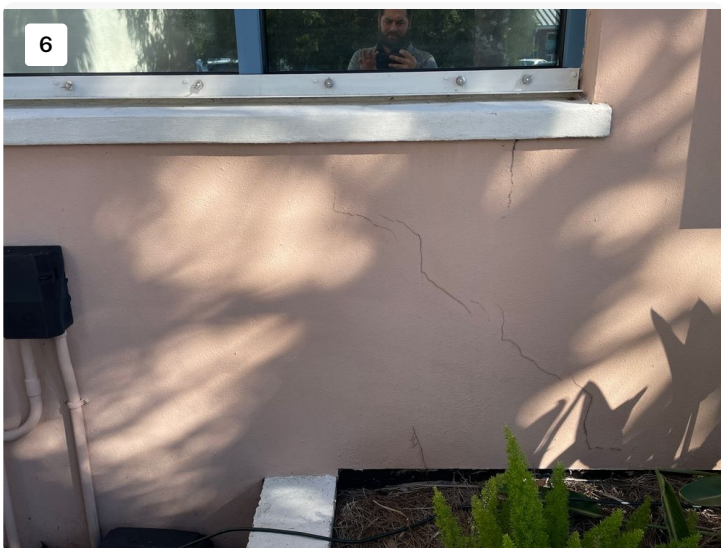
Cracking stucco below windows
