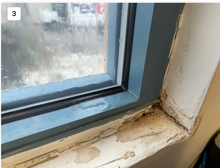
Water test showing water intrusion at windows around window seals and mullion entry points
