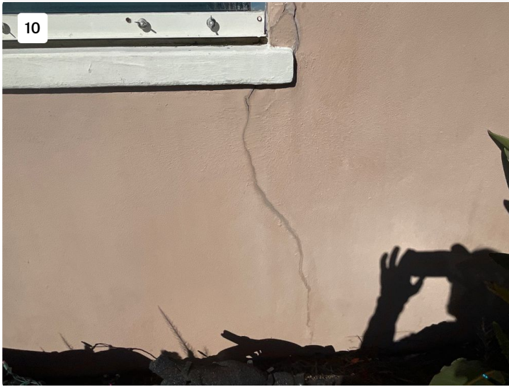
Cracking below window frame
