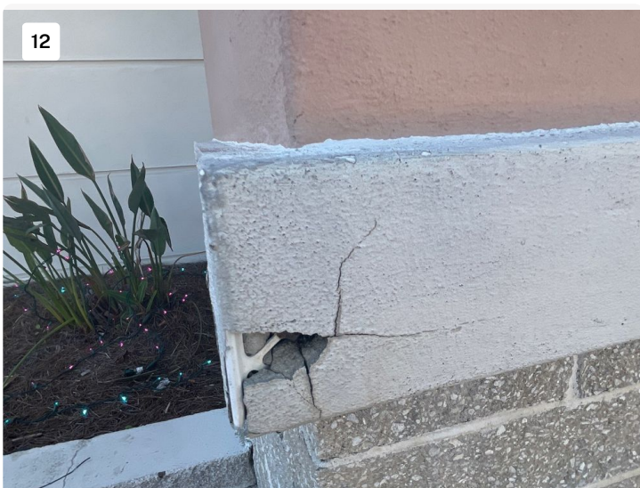
Cracking at pillars
