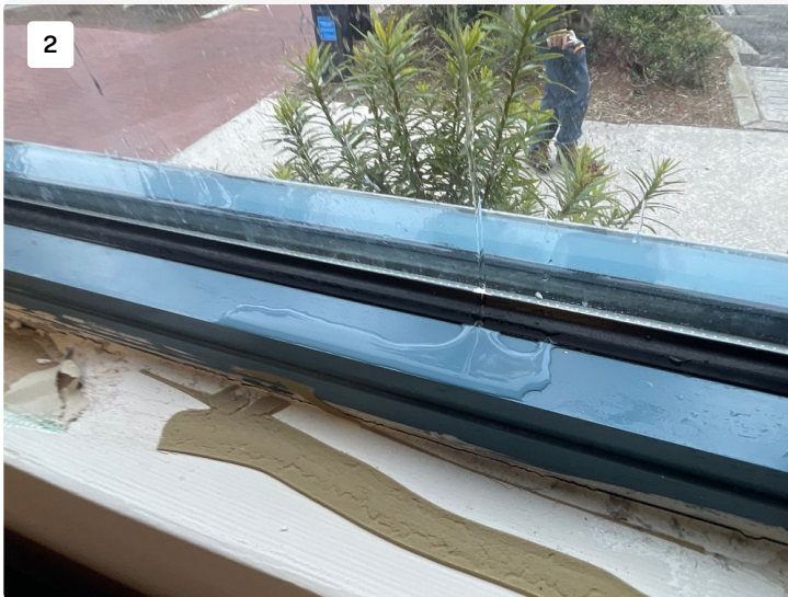
Water test showing water intrusion at windows around window seals and mullion entry points
