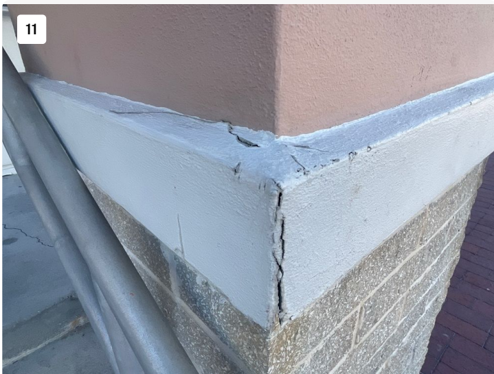
Cracking at pillars
