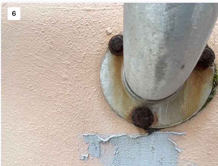
Remove and replace up to 50 bolts in stucco with stainless steel bolts for railings
