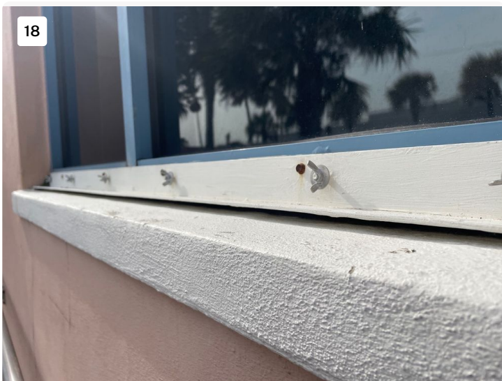
Hurricane shutter braces will need to be removed and reset to properly seal window
