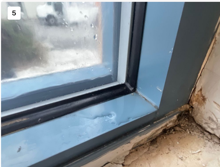
Water test showing water intrusion at windows around window seals and mullion entry points
