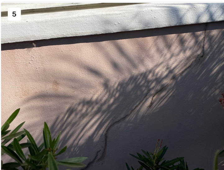
Cracking stucco below windows
