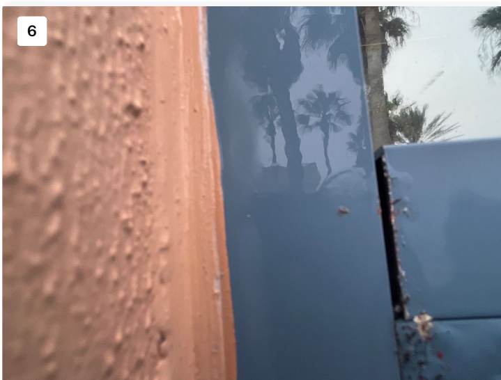
Water test showing water intrusion at windows around window seals and mullion entry points
