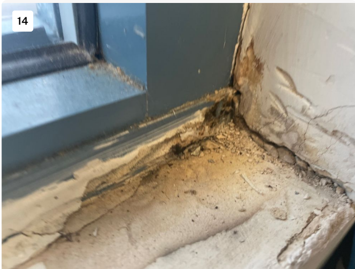
Interior window sill damage
