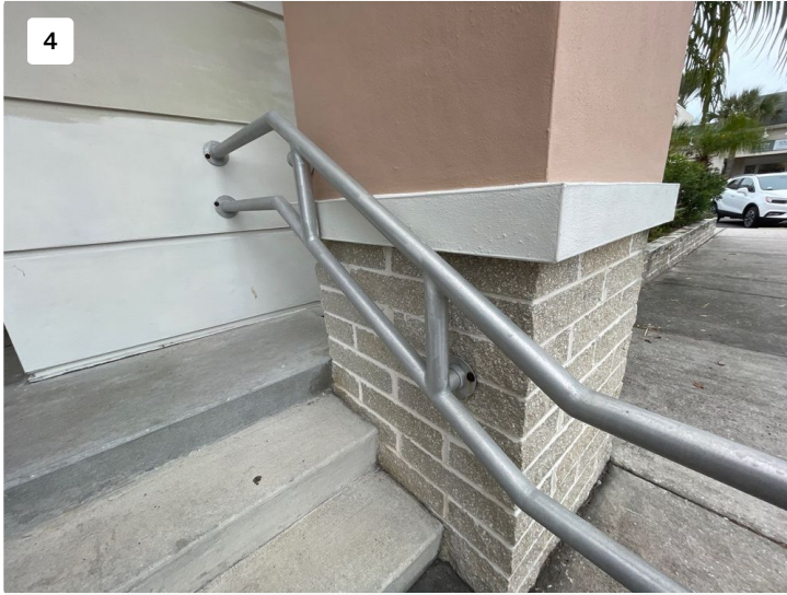
Remove and replace up to 50 bolts in stucco with stainless steel bolts for railings
