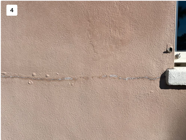
Cracking stucco and bubbling paint
