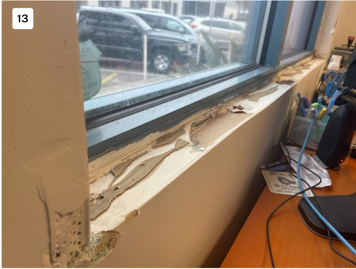
Interior window sill damage
