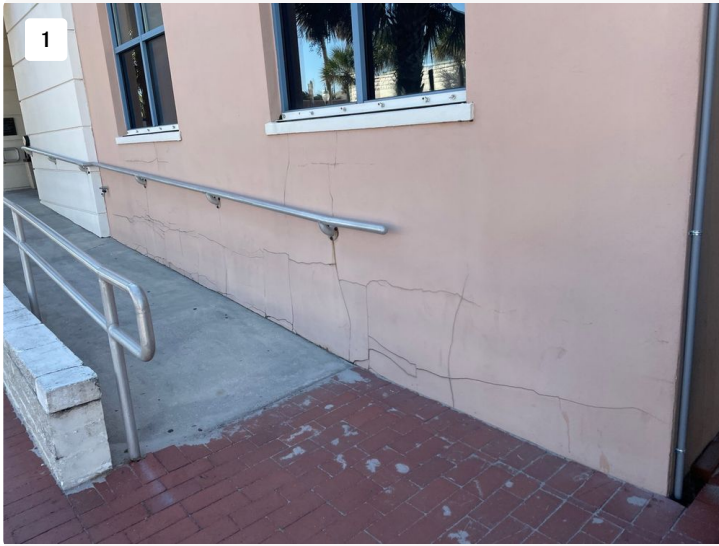
Major stucco damage
