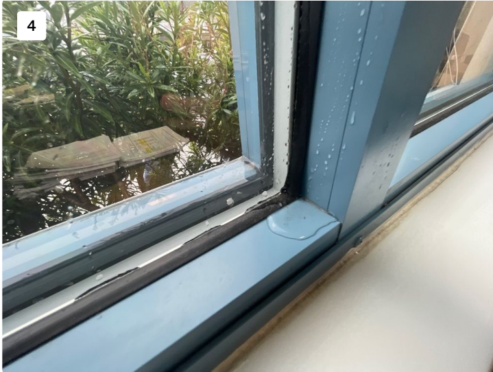
Water test showing water intrusion at windows around window seals and mullion entry points
