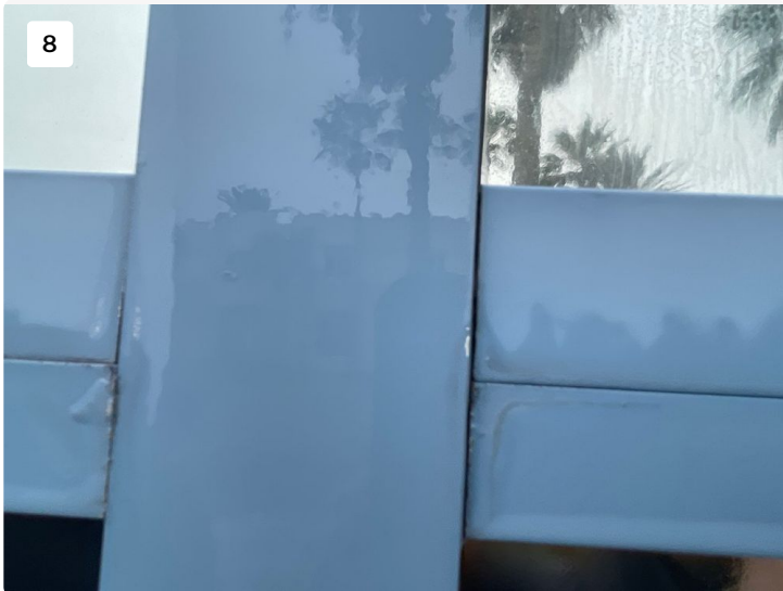
Water test showing water intrusion at windows around window seals and mullion entry points
