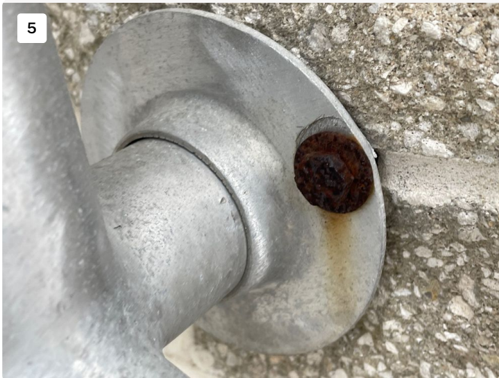
Remove and replace up to 50 bolts in stucco with stainless steel bolts for railings
