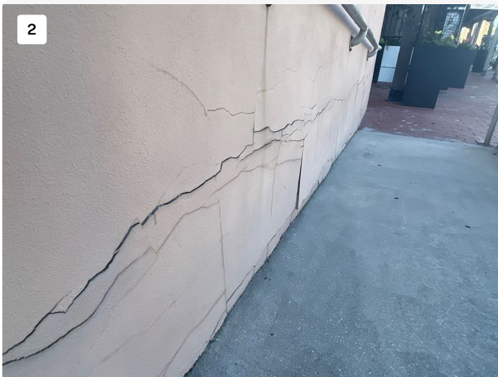
Handicap ramp stucco damage
