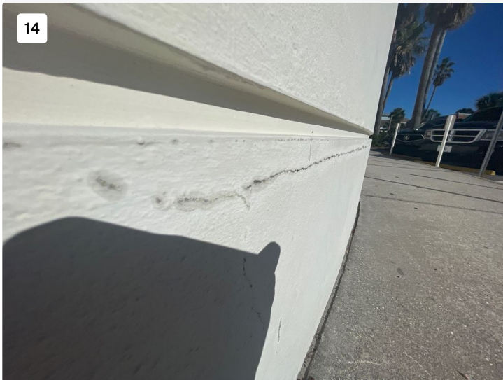
hairline cracking in stucco
