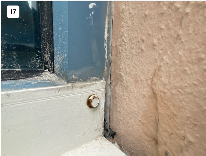
Hurricane shutter bracing directly fastened into aluminum frame and not sealed
