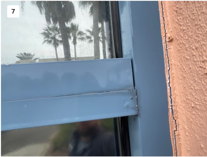
Water test showing water intrusion at windows around window seals and mullion entry points
