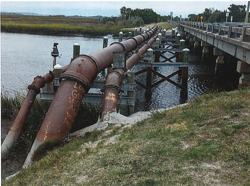
Combined Beaches 12" and 24" Effluent Force Mains at the Sherman Creek (View to North)
