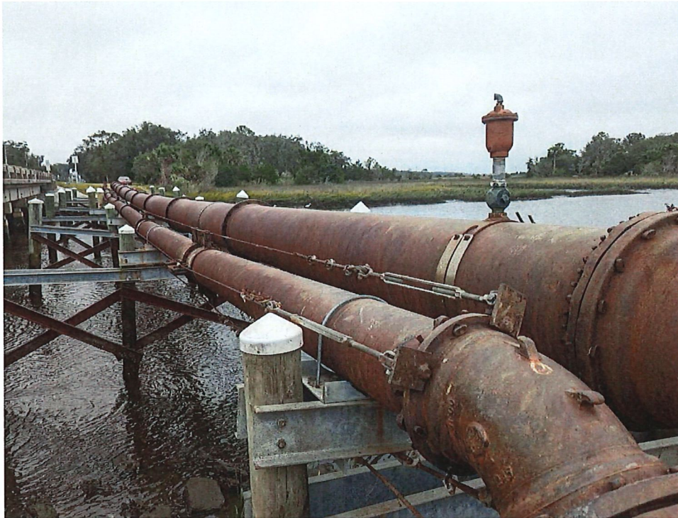
Combined Beaches 12" and 24" Effluent Force Mains at Sherman Creek (View to South)
