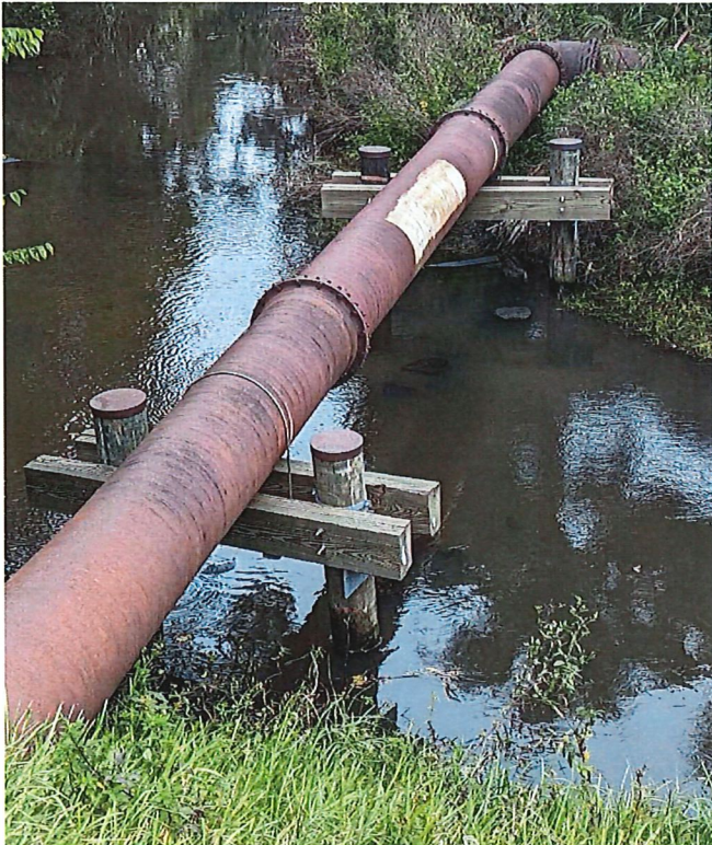
Combined Beaches 24" Effluent Force Main crossing – Sherman Canal @ Mayport Rd
